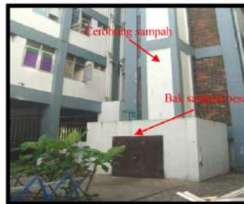
Gambar 5.29 Foto Cerobong/Shaft Sampah R
